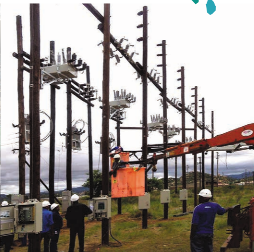
▲ 27 kV outdoor substation with automatic circuit reclosers
