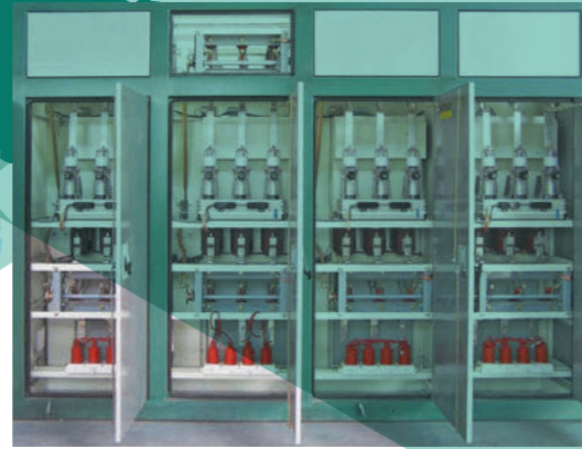
▲ T-Good Electric container-type switchgears for railways
